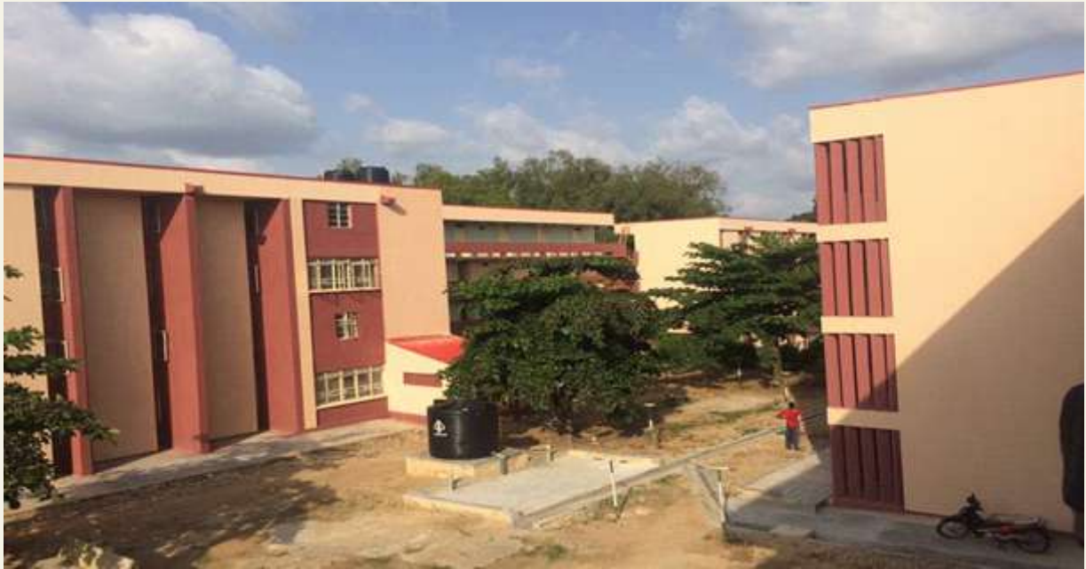
Consultancy for Rehabilitation of Amina Hall Female Hostel Ahmadu Bello University Zaria.
