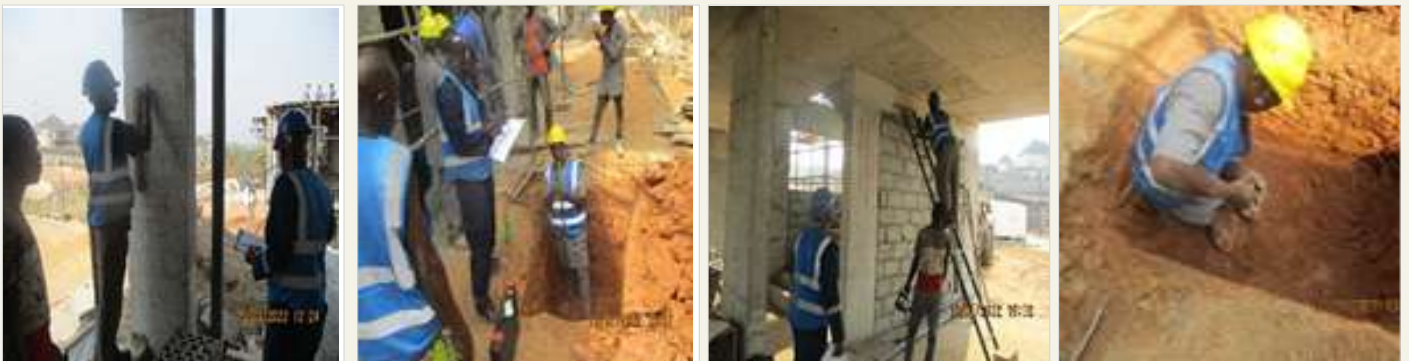
Testing and Certification of Structural Stability of Existing Buildings in Plot 4079 Central Zone A04 Asokoro District Abuja for Sunrise Estate Development Ltd.
