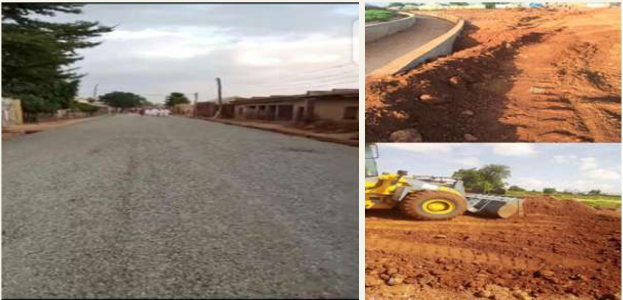
Consultancy Flood Control & Road Improvement Works in JEGA, LGA Kebbi State Project
