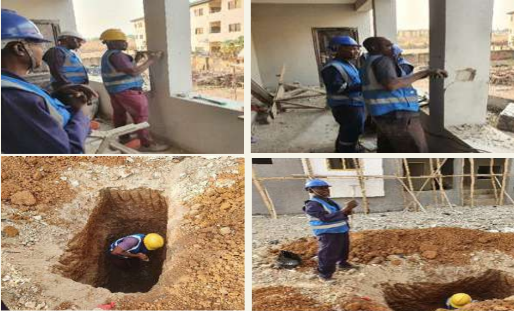
Testing and Certification of Structural Stability of Existing Buildings in Plot 3749 Cadastral Zone E05 Aviation Villa District Abuja for Nigeria Customs Service.
