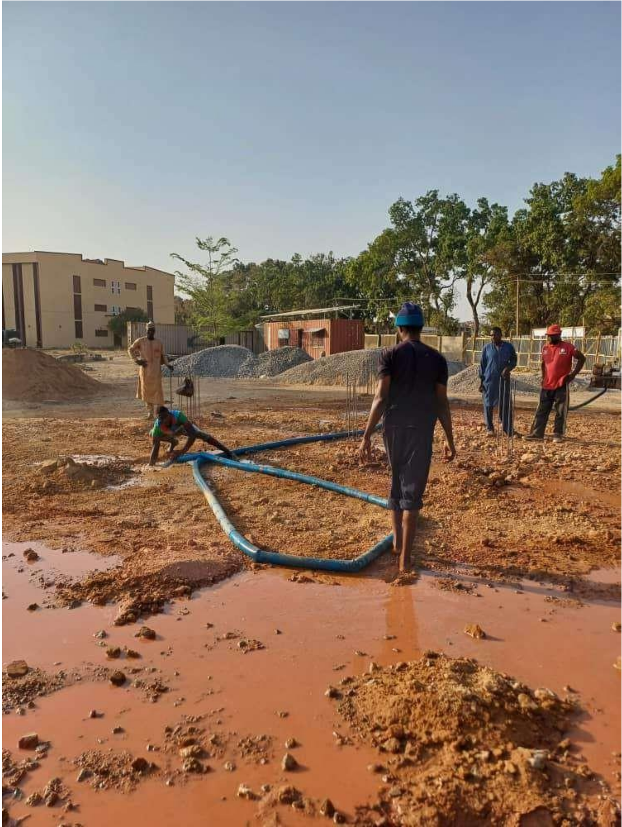
Ponding after Backfilling
