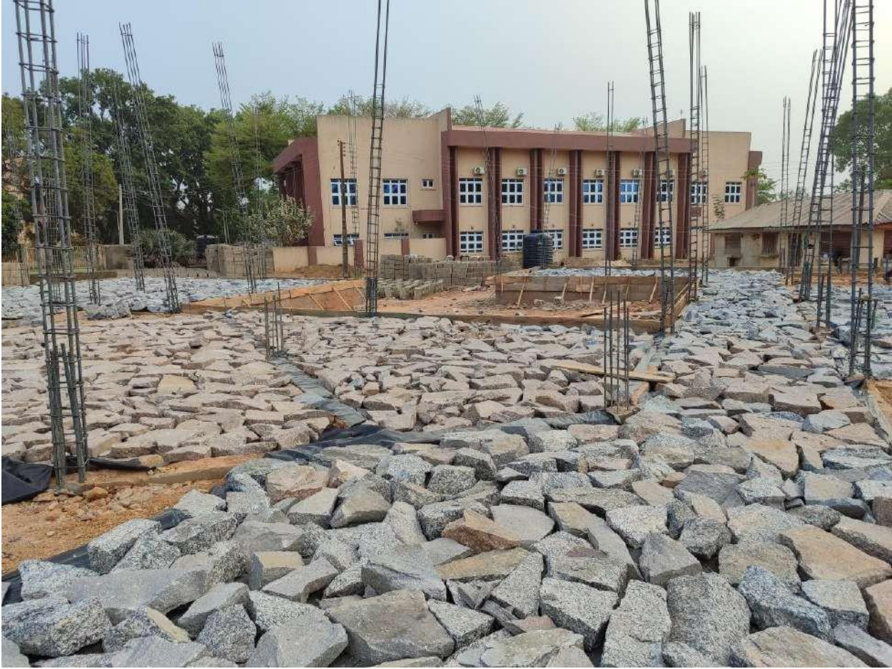
DPM, Hardcore and Formwork placed ready for wire mesh and concrete work
