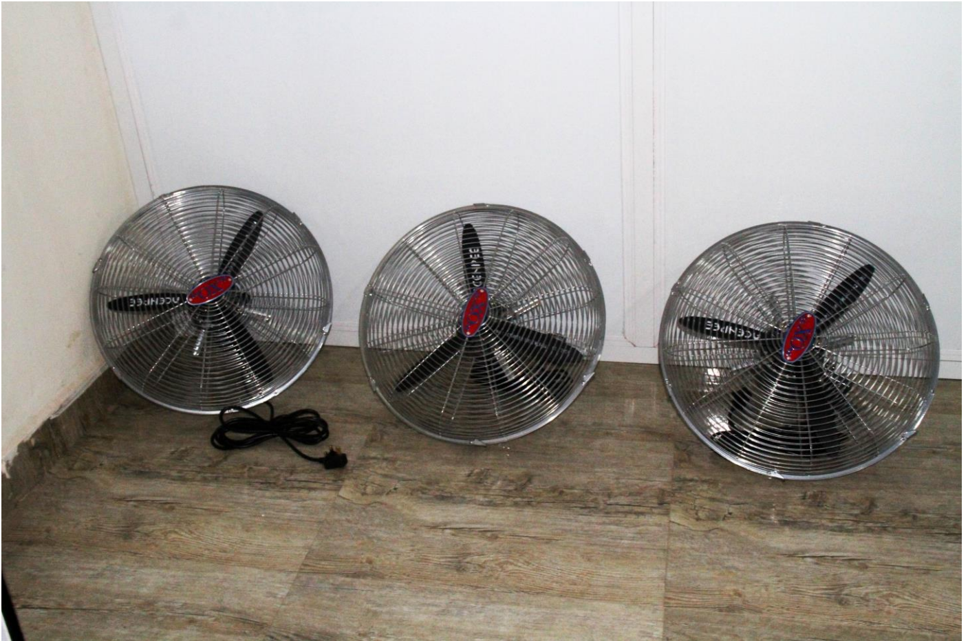
3 Number Office Wall Fans
